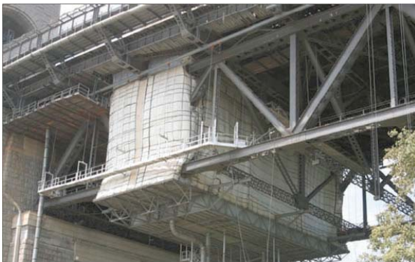
A specially constructed, moveable gantry is used by workers for painting underneath the bridge
