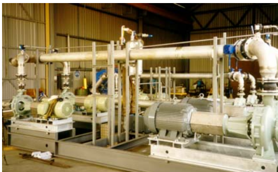
Water pump skid
