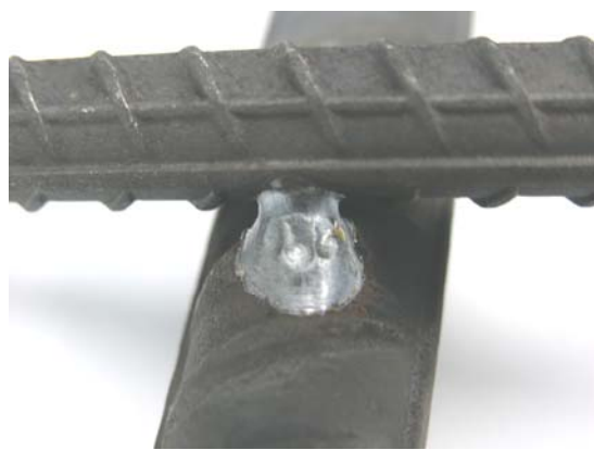
Figure 7. Example of Unacceptable Tack Weld Insufficient weld length
