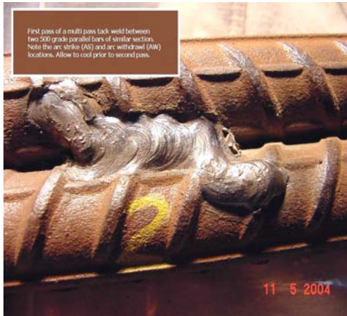
Figure 4. Example of Acceptable Tack Weld Uniform weld geometry
